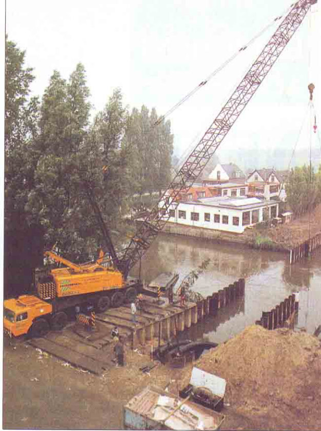
A 58 metre long pipeline being lowered into a pre-prepared trench by a Demag TC-500 truck crane. Slings are attached to both ends of the pipe and to the middle.
